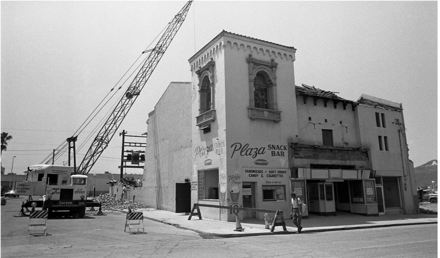
Figure 34. Photograph showing the intersection of Congress Street and Court Avenue during the early phases of urban renewal, looking southwest. C. 1969. Courtesy of Barrio Stories.
