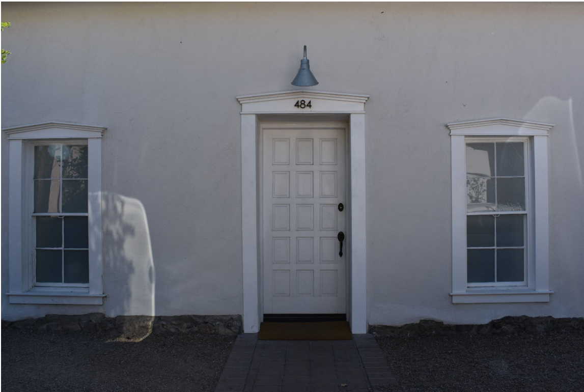
Figure 51. 484 South Convent Avenue showing elements of the Neoclassical style on a vernacular Transformed Sonoran residence. The style is most obvious in the peaked molding that caps all three apertures which is suggestive of a classical pediment. May 2020.
