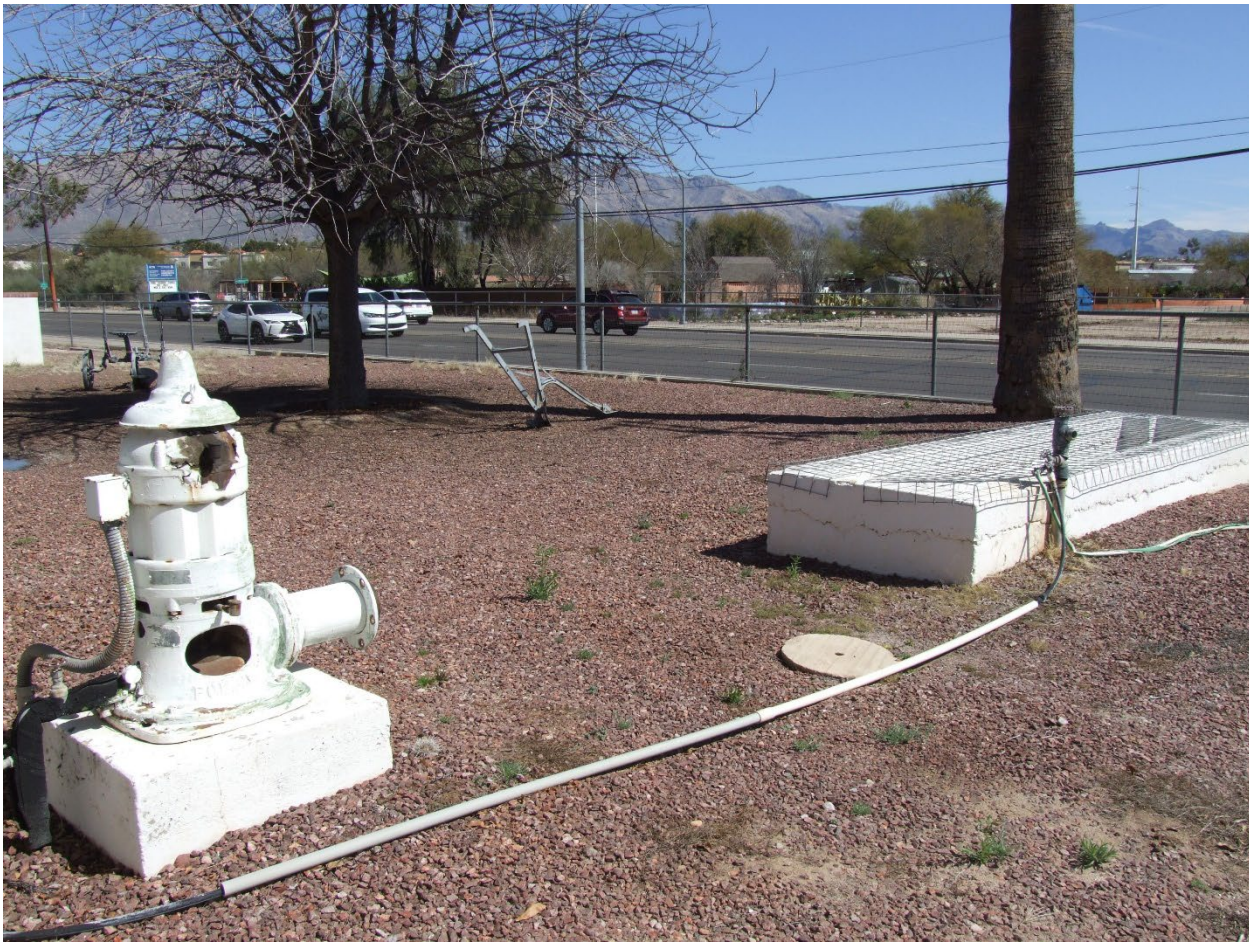
The University of Arizona Agricultural Center, Details of water pump and water holding tank, view facing northeast. WestLand Resources, Inc., March 8, 2023.
