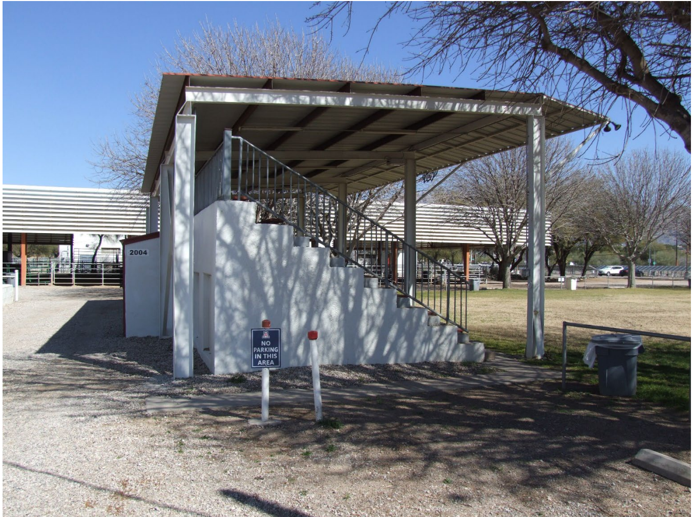
Photograph 27. South elevation of Grandstand; view facing north-northeast (AZ_Pima County_UA Campus Agricultural Center Historic District_0027).
