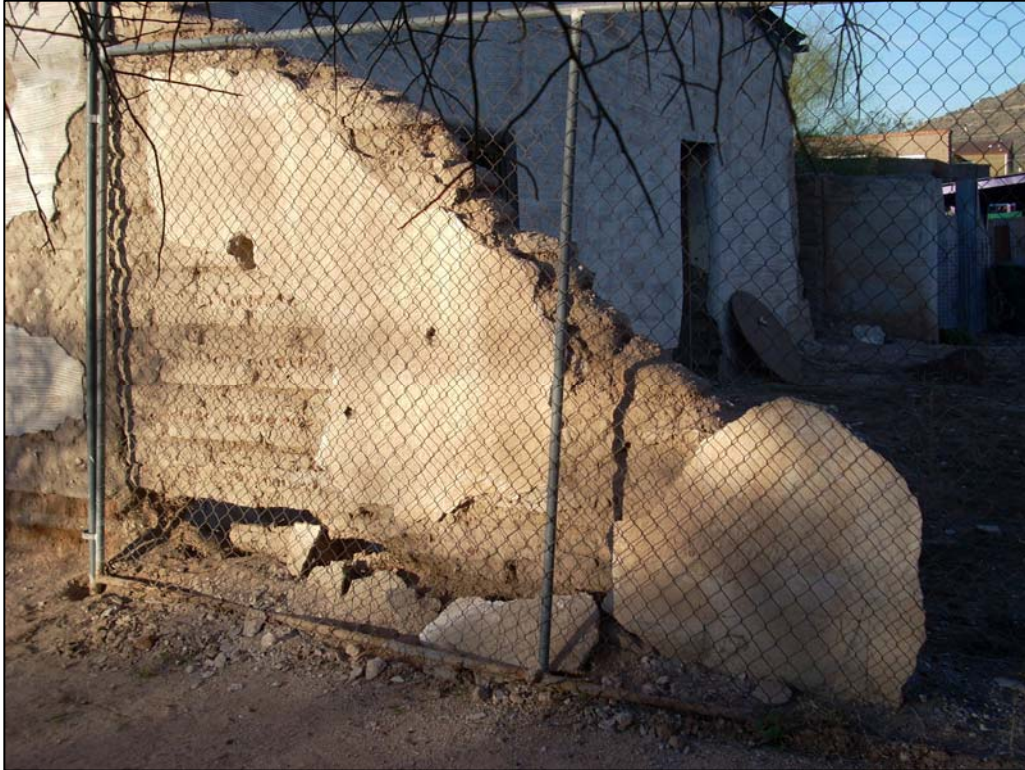
Photo 8. Remnant wall at north end of 576 W. 8th Avenue house; possibly from an extension of the building that housed addresses 566 and 568 S. 8th on the 1909 Sanborn map.
