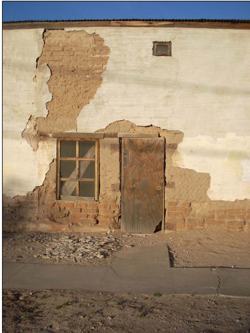
Photo 17. The house at 576 S. 8th Avenue, showing recently applied cement plaster in a state of deterioration.
