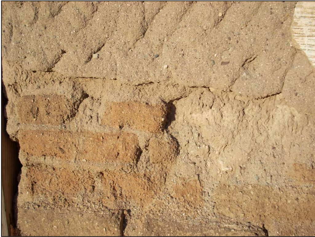
Photo 16. Detail of exposed adobe bricks beneath mud plaster at the house at 576 S. 8th Avenue house; view to the west.
