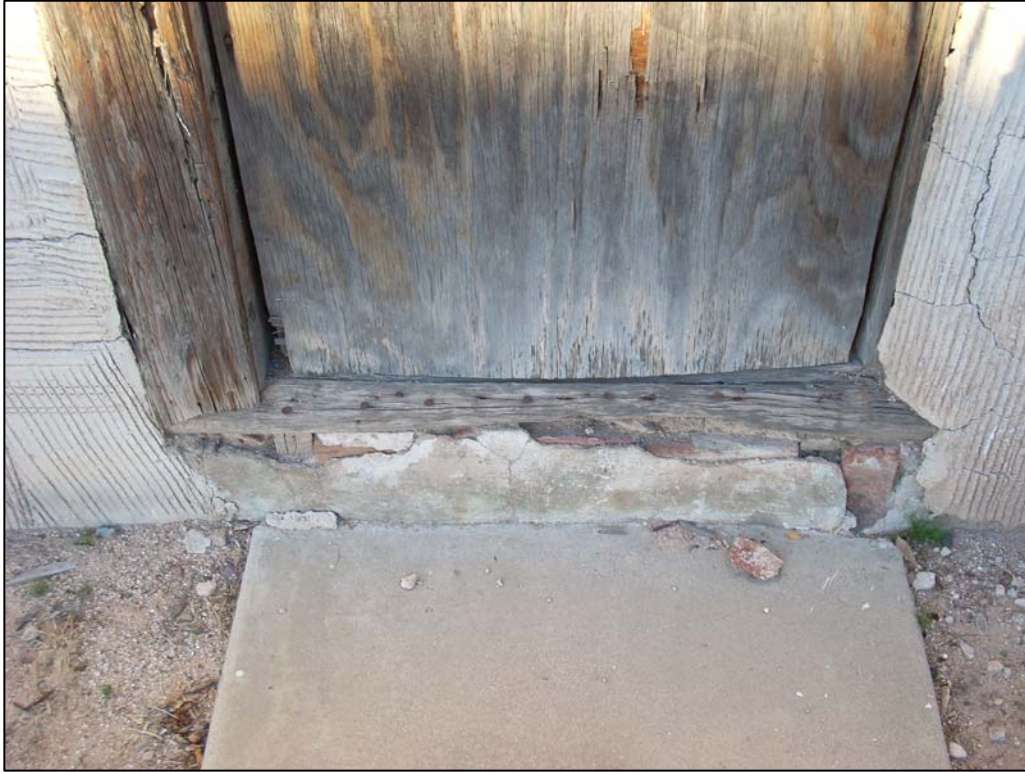
Photo 14. Detail of elevated brick/lumber threshold of the doorway of the house at 586 S. 8th Avenue.
