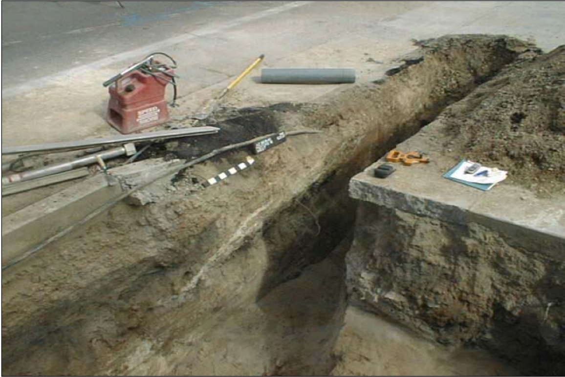
Photo 29. Feature 18, portion of excavated area; view is downward and to the northwest.
