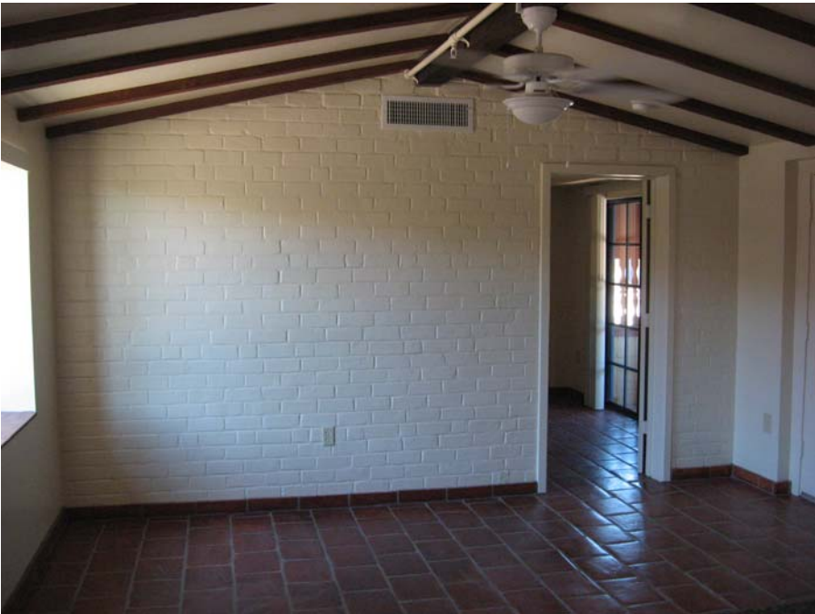
37. Original Building Group Typical livingroom looking into bedroom infill of a carport at a rehabilitated Joesler-designed duplex. Brick wall, roof beams, and tile floors are preserved. (Photo by Don W. Ryden of Ryden Architects, Inc., 2010)
