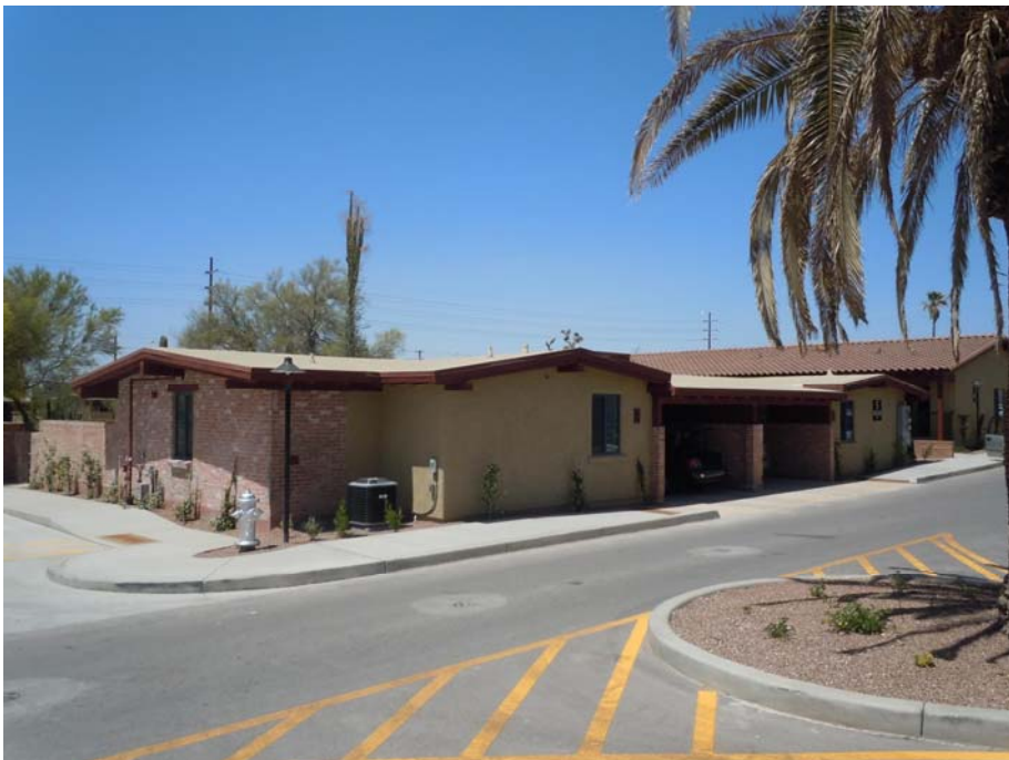
27. Second Building Group Addition Contemporary Style duplex (Building P) with rear addition and original carport. View to northwest. (Photo by Don W. Ryden of Ryden Architects, Inc., 2011)
