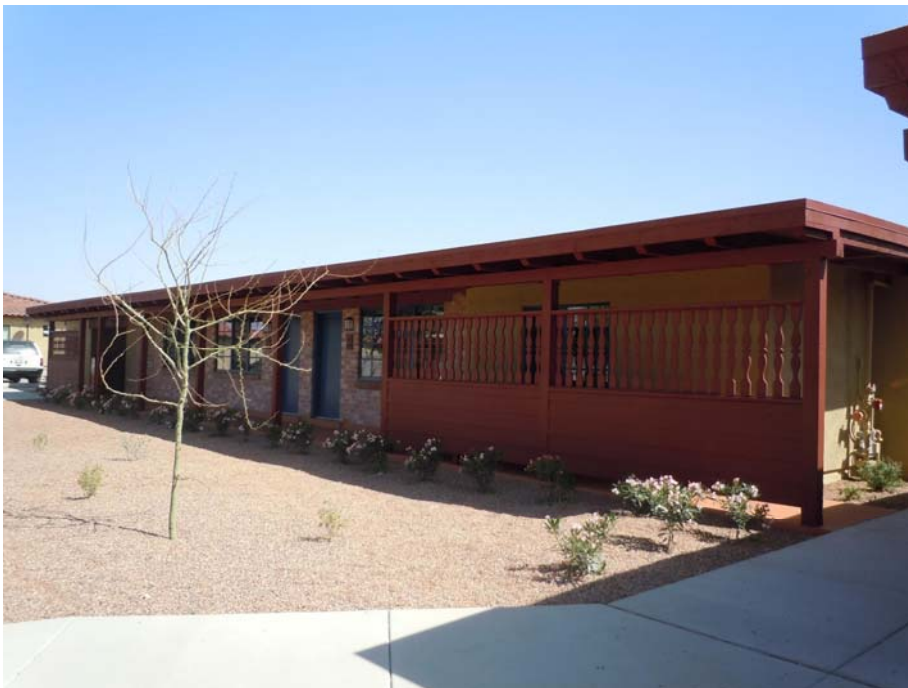
18. First Building Group Addition Spanish Colonial Ranch Style linear units (Building I) with covered walkway and end carports. View to southeast. (Photo by Don W. Ryden of Ryden Architects, Inc., 2011)
