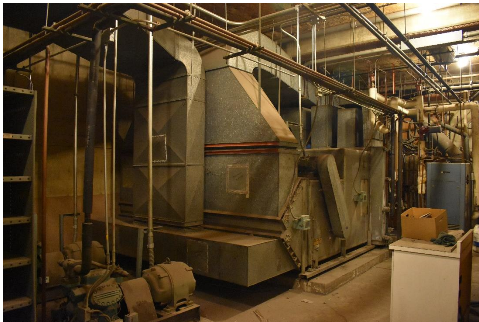
Figure 14. ASARCO Headquarters, showing basement boiler, looking southwest (Logan Simpson 2021 [AZ_PimaCounty_ASARCOHeadquarters_0012]).
