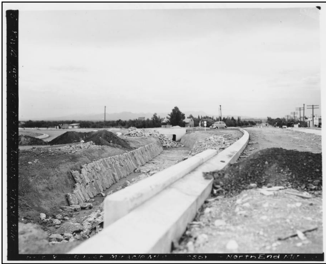
1937 Miracle Mile improvements under construction. (Arizona Historical Society/Tucson AHS Photo Collection 180 F103 54)
