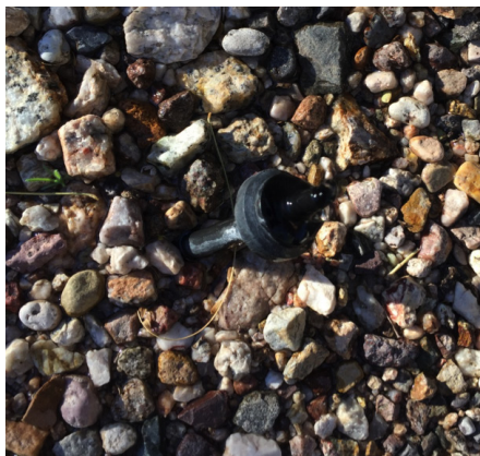
This drip emitter is connected to micro-tubing which is attached underground to a lateral line..
