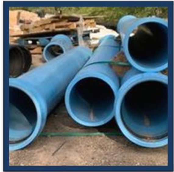
Figure 13: Wet Utility Pipes
