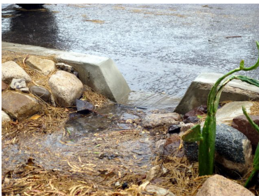
Curb cuts allow stormwater runoff to enter a landscaped basin in the public right of way (Photo credit: Watershed Management Group)
