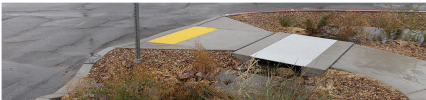
Image 6.5 A sidewalk scupper in a curb Credit: Watershed Management Group
