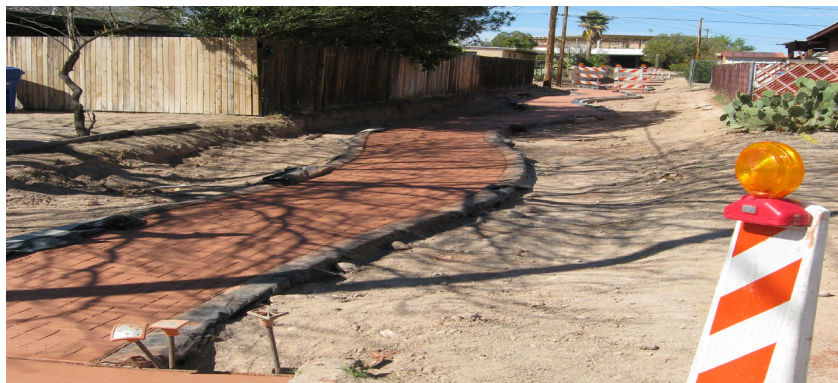
Image 6.7 A green, pervious alley being constructed in Sugar Hill Credit: Watershed Management Group
