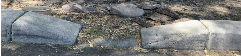
Image 6.2 A curb inlet conveys water off the street
