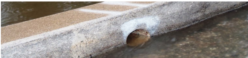
Image 6.4 A curb core with flowing water Credit: Watershed Management Group
