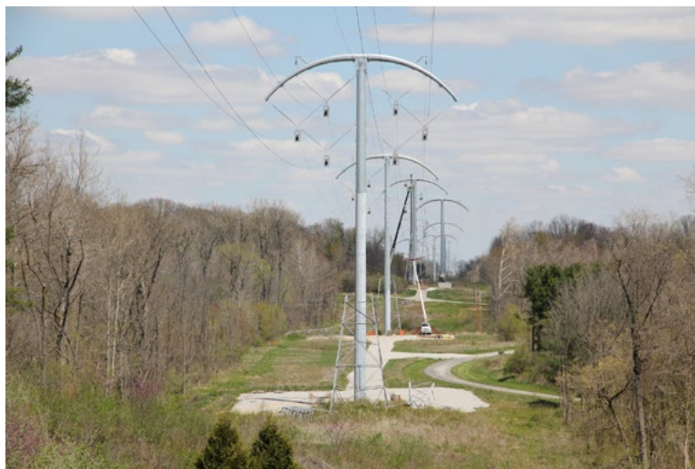
Figure 15.—Robison Park-Sorenson project during construction. Photo by BOLD Transmission, used with permission.
