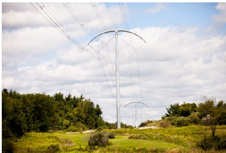
Figure 14.—Robison Park-Sorenson simulation of BOLD design. Photo by BOLD Transmission, used with permission.
