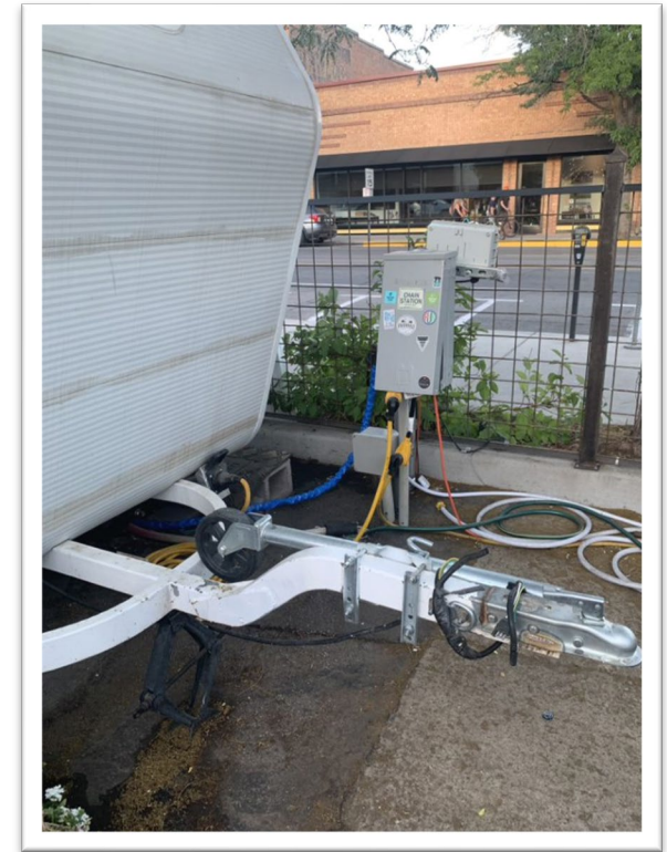
Permanent Power Pedestal Example
