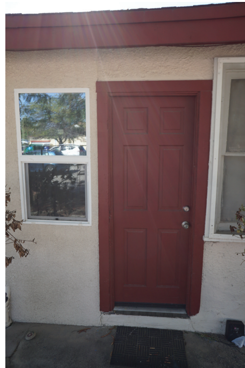
REPLACED ORIGINAL: WOOD SINGLE HUNG, 1/1 NEW: VINYL SINGLE HUNG, 1/1 DOOR IS EXISTING, NOT REPLACED
