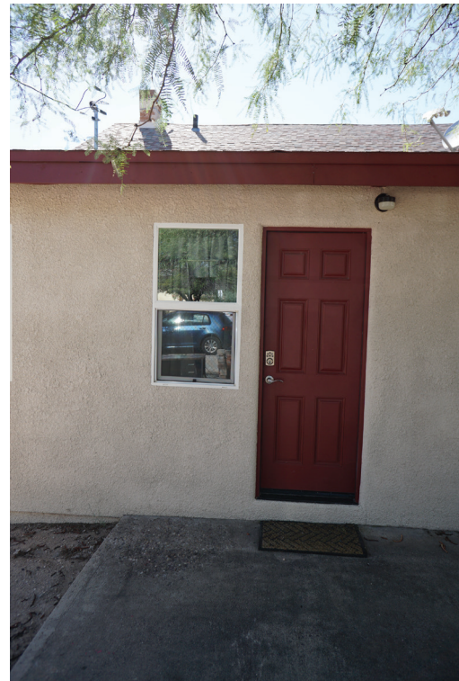
REPLACED ORIGINAL: WOOD SINGLE HUNG, 1/1 NEW: VINYL SINGLE HUNG, 1/1 DOOR REPLACED ORIGINAL: WOOD NEW: WOOD
