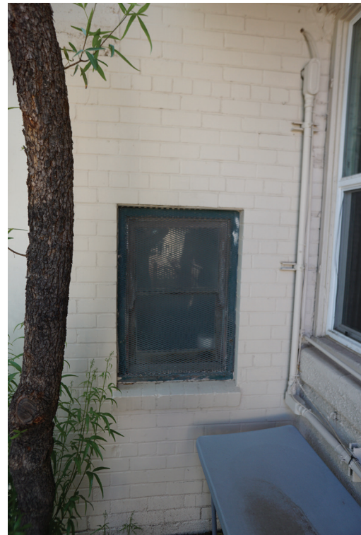
EXISTING NOT REPLACED
