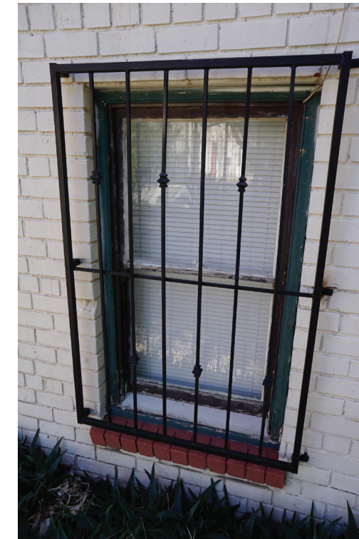
EXISTING NOT REPLACED
