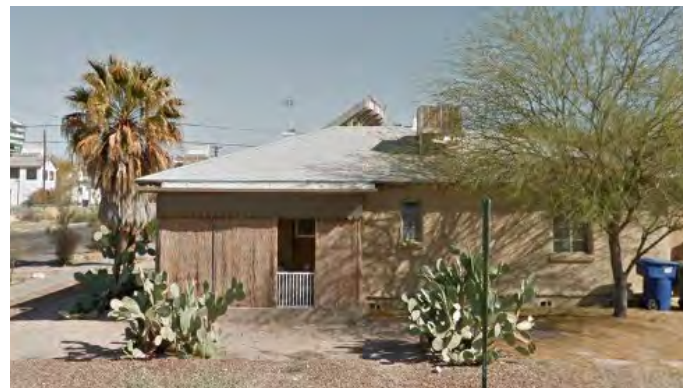
Enclosure has altered the character-defining porch and risks a loss of integrity.
